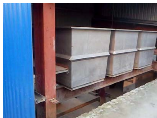
Latex Reception Tank
